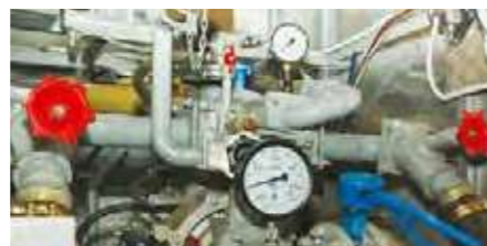
Pump and valve control
