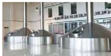
Brewery production equipment
