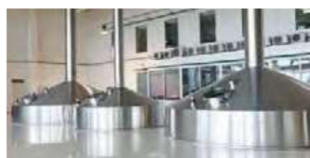
Brewery production equipment
