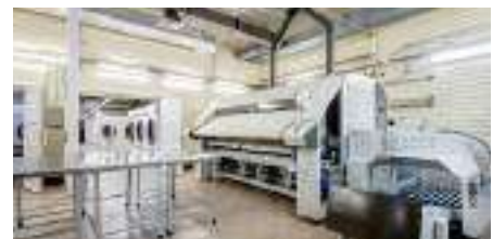
Automated laundry system
