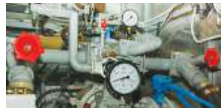
Pump and valve control
